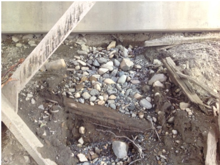
fill ravelling under ballast wall on left bank
