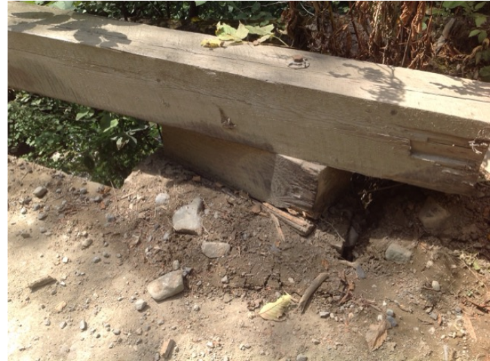
guardrail off riser
